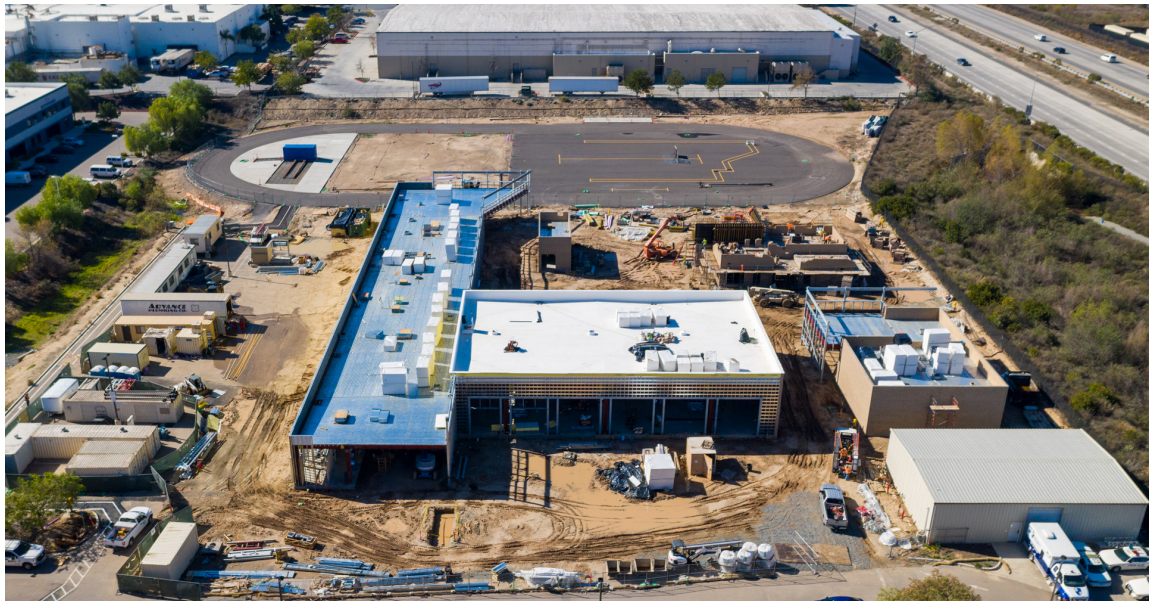
The Public Safety Training Center at the Higher Education Center at Otay Mesa is taking shape.
